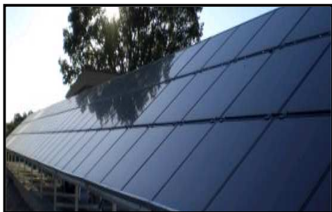
In 2010, Chile will be home to the 1 st photovoltaic plant in South America; located between San Pedro de Atacama and Toconao.
